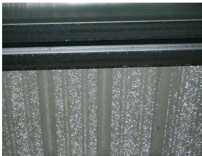
Fig. 4: Condensed water on the inner surface of the roof cladding [3]
