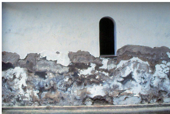
Fig. 1: Surface layer destroyed by moisture and salts
